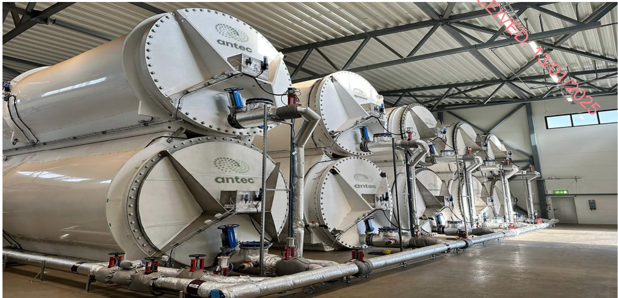
Plate 1: Typical Reactor Bank
